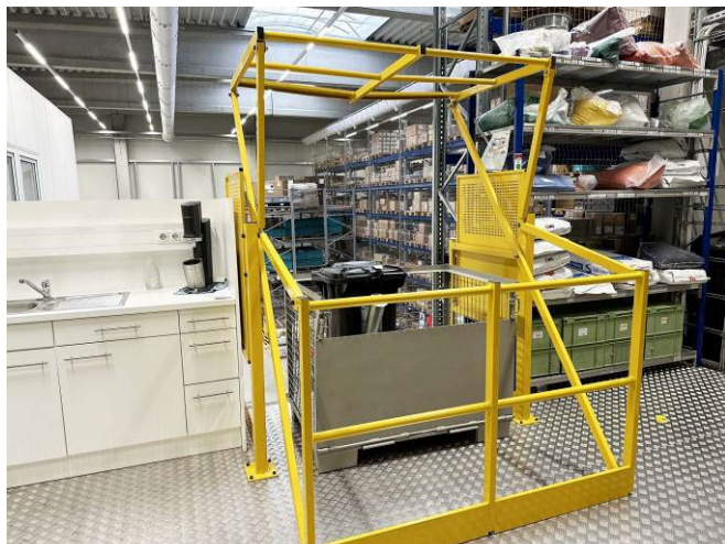
Fig. 3: The material bin filled with granulate is lifted to the upper floor towards the central materials handling system, using a fork lift with sophisticated safety devices.
